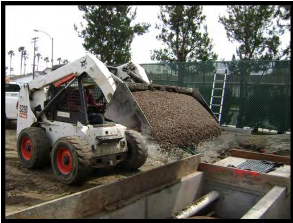
Approximately 8.5 Cubic Yards of Filter Media Are Carefully Placed Into The Modular Wetland
