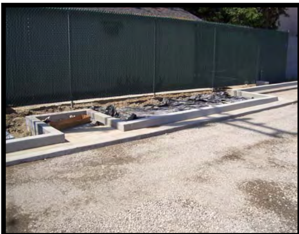
The Curb And Gutter are Pored And The Site if Ready for Pavement
