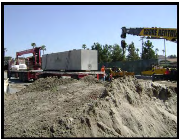
Delivery Truck Is Positioned To Off Load Modular Wetland With The Crane Standing By (contractor to provide the crane)
