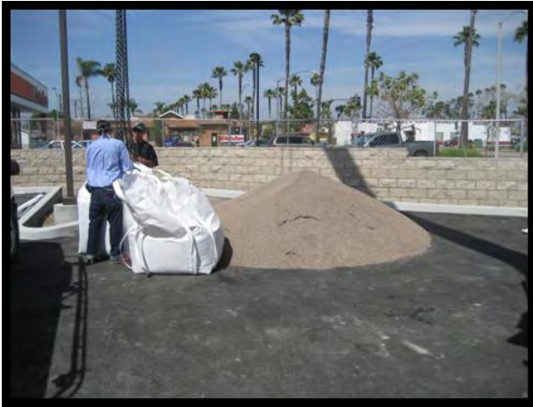
The Delivered Filter Media Is To Be Prepared To Be Washed And Mixed
