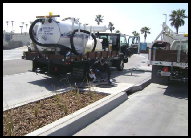
Service Crews Arrive On Site And Remove Access Manhole To Perform Maintenance Service.
