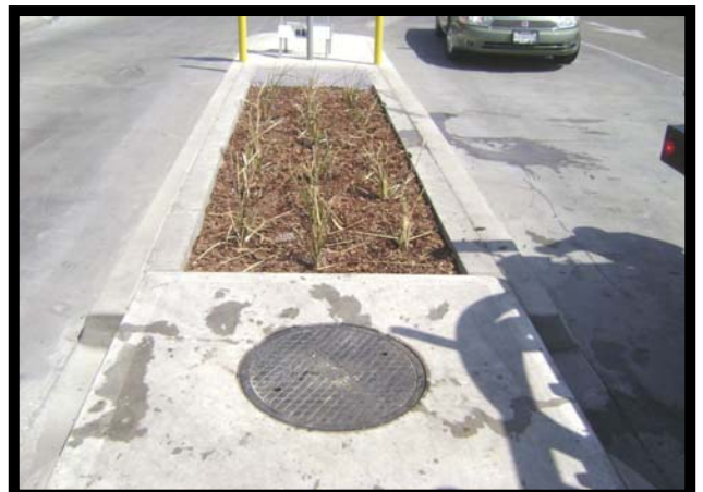
Replace Access Manhole. Check Plants For Growth, Trim If Necessary. Service Is Complete. Total Service Time = 45 Minutes.
