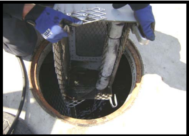
Cleaned Catch Basin Filters Are Removed Through Access Manhole To Allow For Unimpeded Access To Sediment Chamber.
