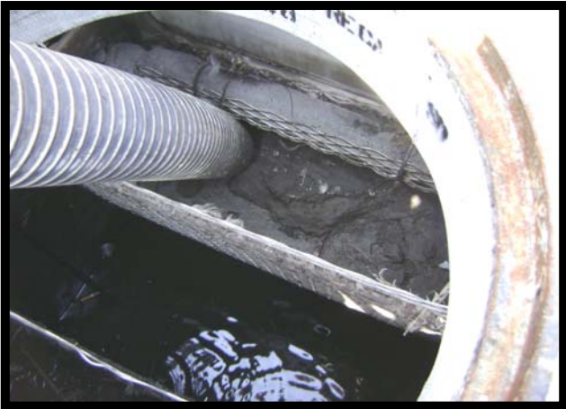
Catch Basin Filters Are Completely Vacuumed Free Of All Pollutants.
